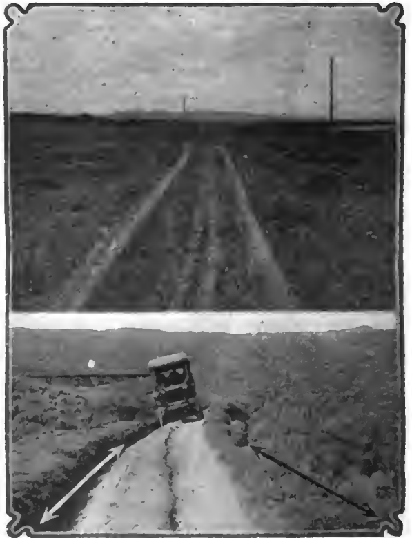
Upper—This shows a section of a 70-mile stretch that does not vary 2 per cent. in grade or character in its distance across the eastern Wyoming plains between Laramie and Medicine Bow, and over what is known as the Laramie plains. Because it is some miles away from the railroad, for more of which distance it is to be abandoned, and a new road is now being finished between the same points, near the railroad for automobile travel. It is on alkali soil and naturally well drained.
